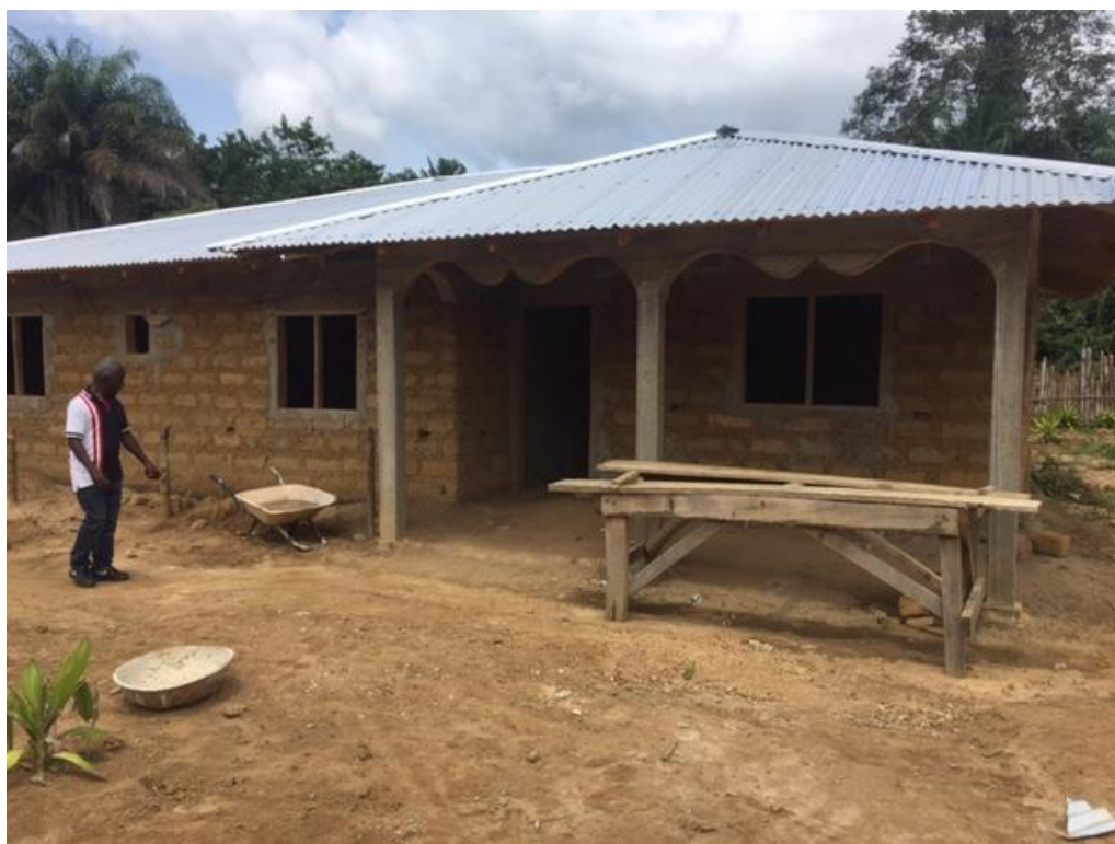
The QIT of Bambalah is building staff quarters near the clinic which includes 2 rooms for pregnant mothers.
