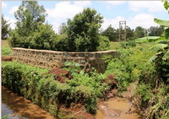
Fig. 6. Retaining wall constructed to minimize contamination and ensure safe water is available during flooding.
