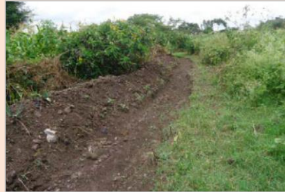
Fig. 7. Diversion ditch constructed to protect the source water for a community of over 6000 inhabitants from the Ellie kebele. Indigenous tree planting complimented this activity to protect and maintain the water table.
