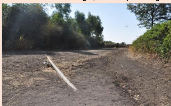
Fig. 4. Exposed main supply pipelines as a result of heavy rainfall/flooding were commonly found in piped water supply systems, representing a significant risk to water safety and availability.
