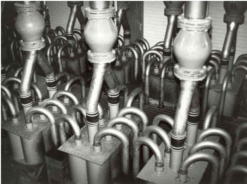
Figure 5. Multistage pressure swirl concentrators specially designed by Seppo Ryyänen for Pätt wastewater treatment plant. They were in operation from 1985 to 2001. (Häkkinen et al 1987)
